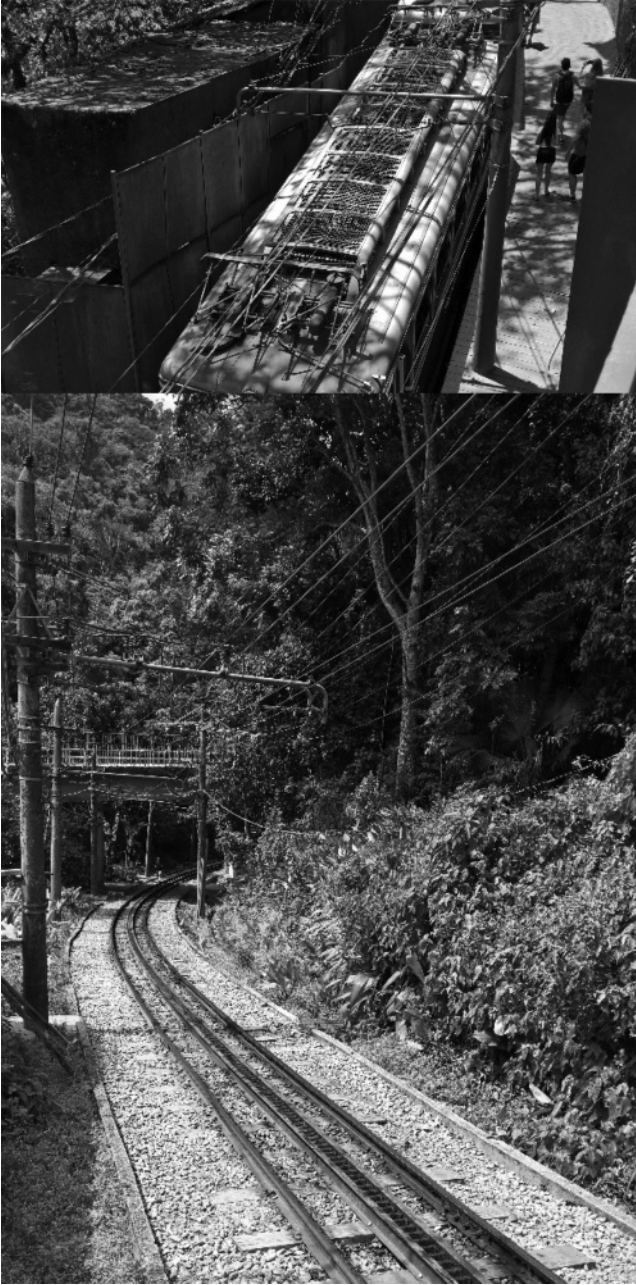
Figure 1.5 Particular three-phase AC railway electrification system at mains frequency for the Corcovado Railway in Rio de Janeiro, Brazil.
