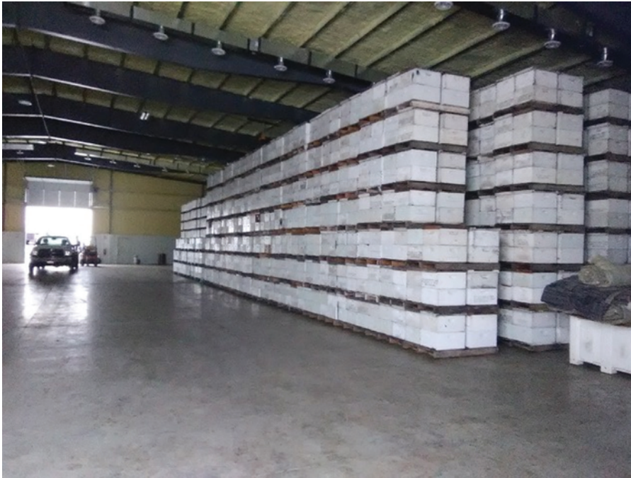
Figure 1.4 Colonies of bees stacked in preparation for overwintering in the indoor storage building. Modern ventilation ductwork is visible in the ceiling. Refrigerated air keeps colonies at 40 °F. Air handlers push fresh air into the building, exhausting higher-level CO 2 outdoors. Source: Photo by John Miller.
