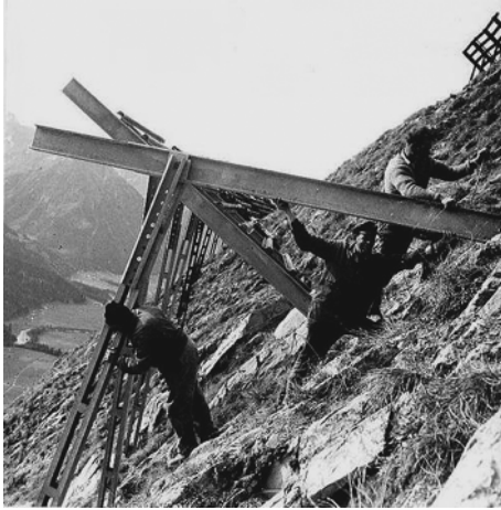
Fig. 1.12 First avalanche defense structures in the starting zone with prefabricated snow bridges in steel, Heuberg, Häselgehr (© WLV Tyrol).
